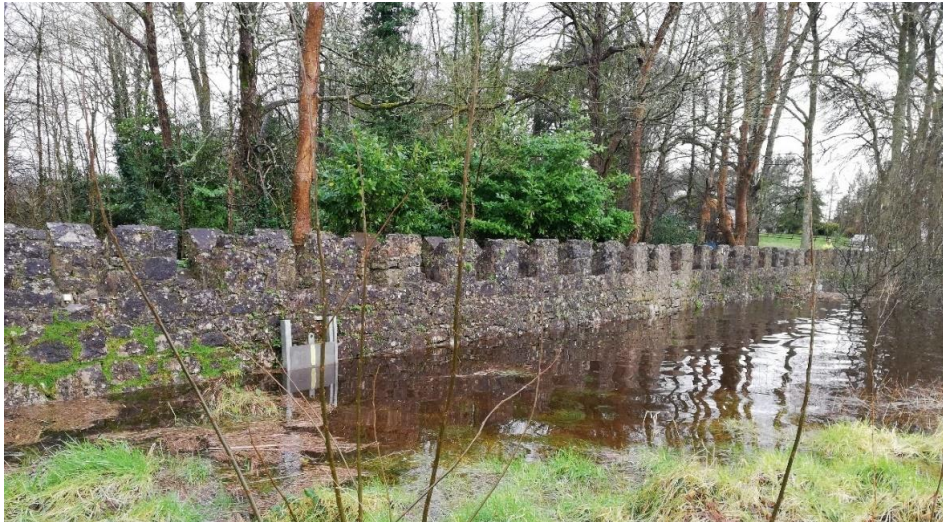
Figure 6-11 One of three sluice gates at Island House Causeway, shut during winter flooding
