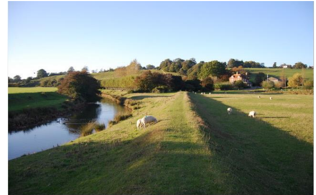
Example of flood embankment (River Tillingham) (Image copyright: N Chadwick under the licence Creative Commons — Attribution-ShareAlike 2.0 Generic — CC BY-SA 2.0 )
